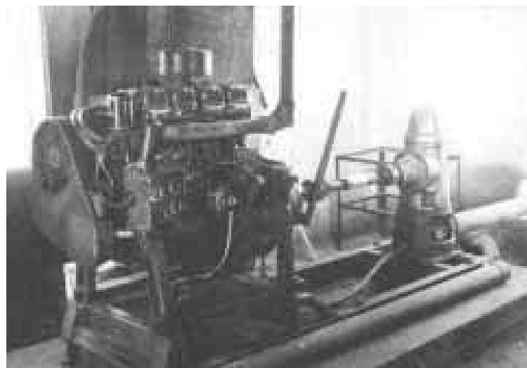
Figure 4: A diesel-powered pumping system
