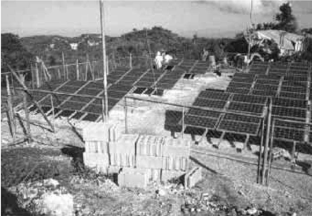
Figure 50: Photovoltaic drinking-water pumping system in the Philippines
