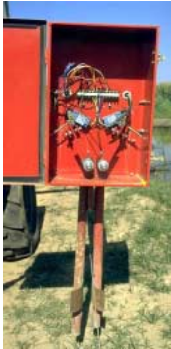
Control of a linear-move sprinkler with a guide wire
